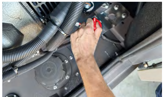
Battery isolator lockable, it is used during maintenance and storage
